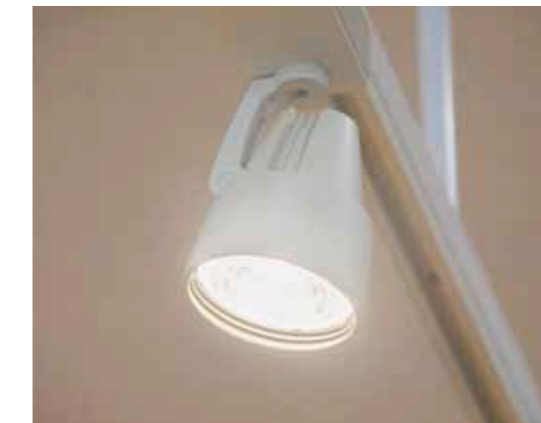
There are other base down lights, a universal down light.
